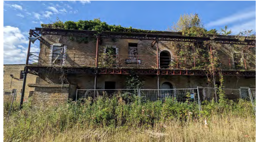
Figure 26 The Barracks are an example of part of the Site which is currently unusable, due to its current condition
