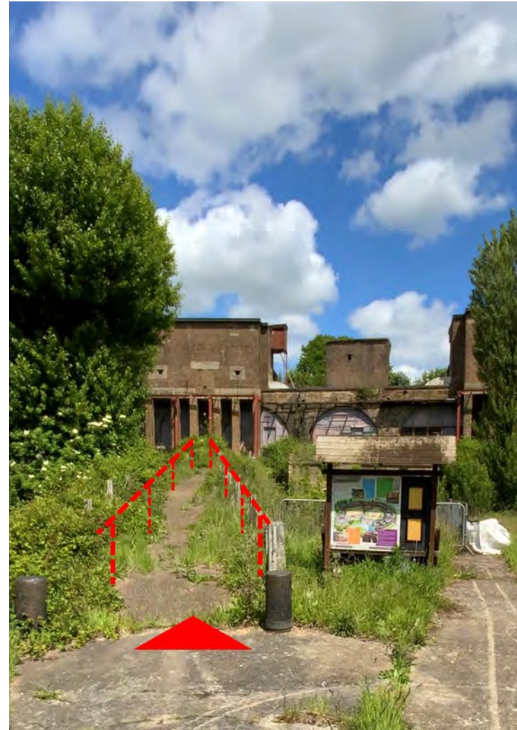
Figure 124 The East Ramp will require repairs to the surfacing and the gradient checking and potentially flattened, together with the provision of intermediate landings and new handrails to both sides to conform to Building Regulations Part M
