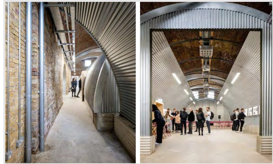
Figure 142 Examples of lining to brick railway arches using corrugated galvanised steel sheet. It may be possible to adopt an approach of installing lining only where required, however this risks ongoing maintenance issues with future leaks that may not currently be evident, and the damp issues at Coalhouse affect the full surface of the vaults
