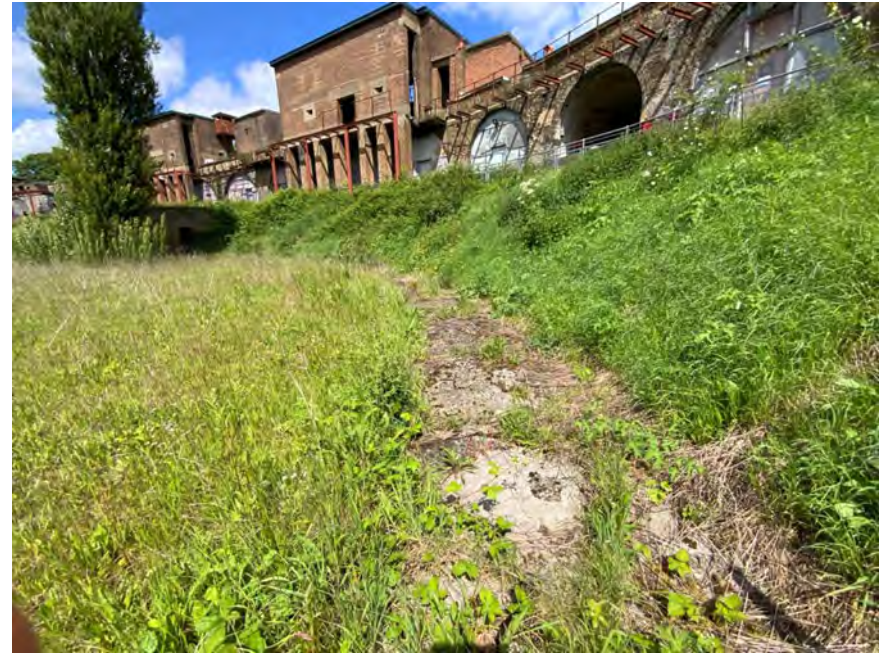
Figure 126 The Parade Ground path will require repairs to the concrete surfacing
