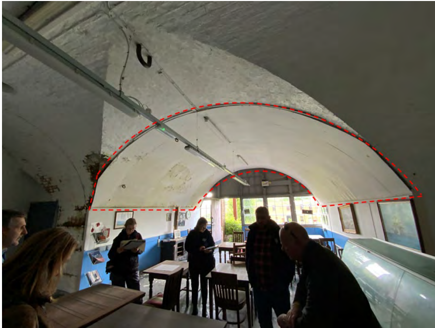
Figure 137 Example of existing lining to vaults; the peeling finishes, staining and 'rippled' surface are as a result of the use of incorrect non-waterproof materials.
